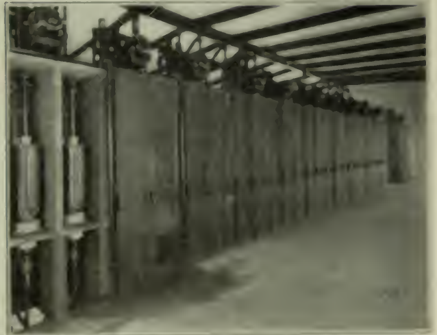
OIL BATTERIES IN TRANSFORMER HOUSE
